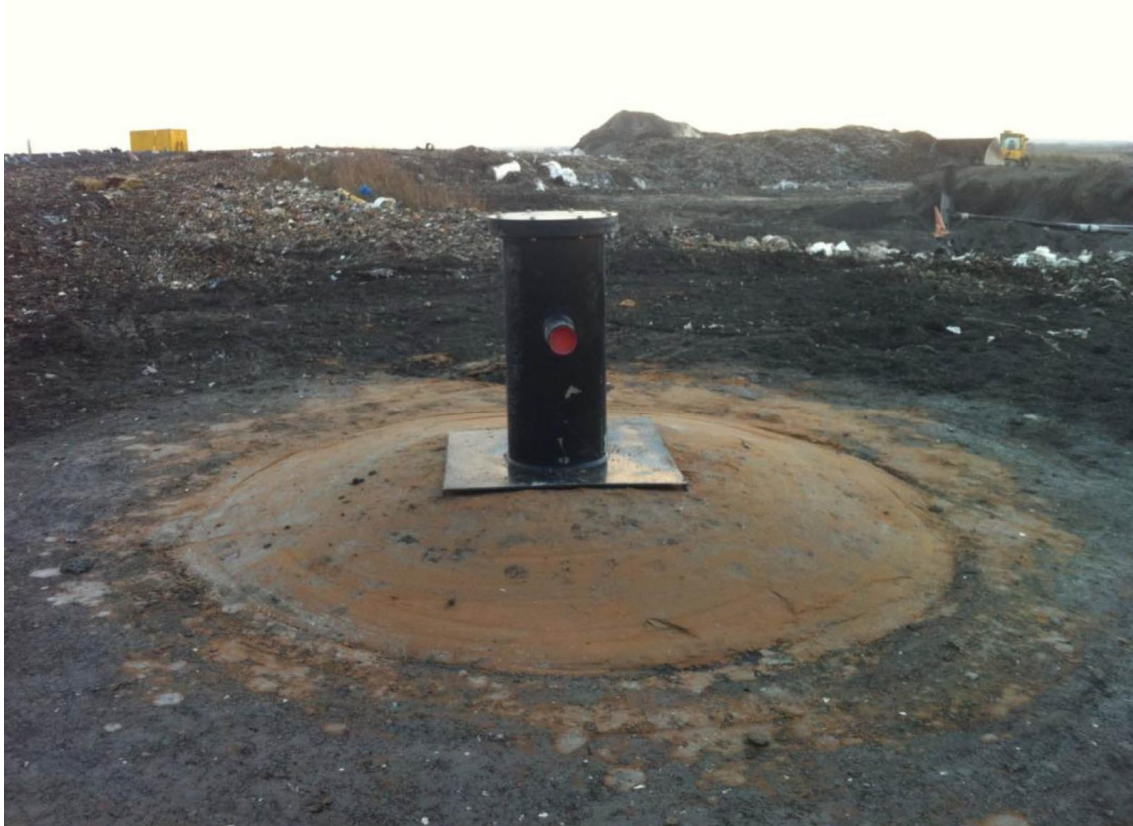
Figure A4-2 Multiwell V-type placed under angel and connected in 1 collector put at landfill Vink
