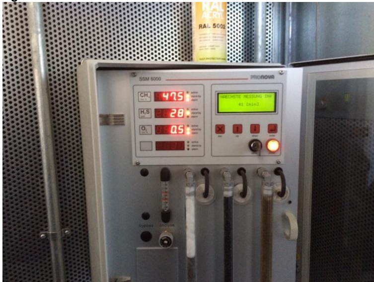
Figure A6-3 Online measurement of extracted LFG landfill Samara
