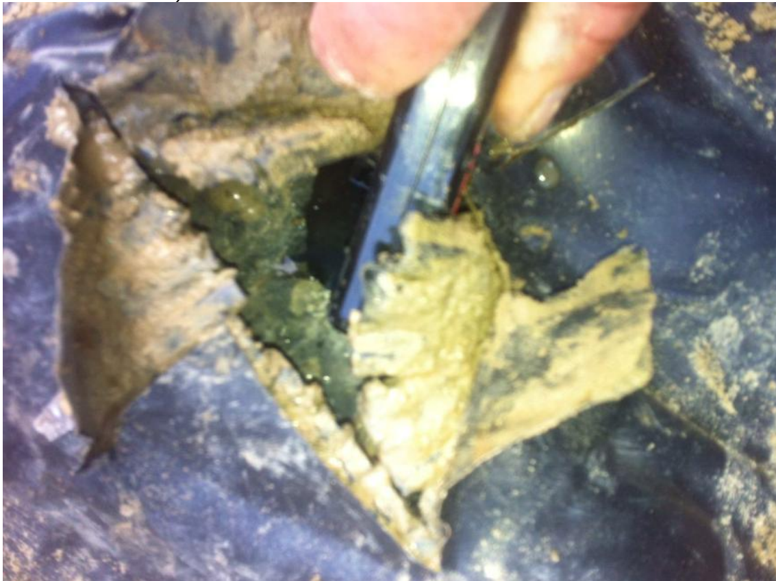
Figure A7-2 Drain collector put at Zabrze landfill Visible wet clayey soil around drain (ribs are 'filled')
